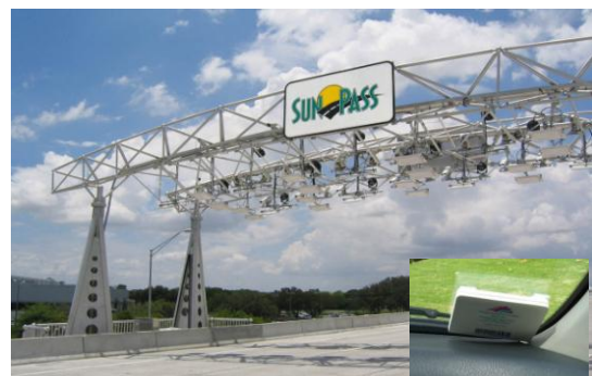
Fig.4. SunPass RFID Tolling and Traffic Control System
