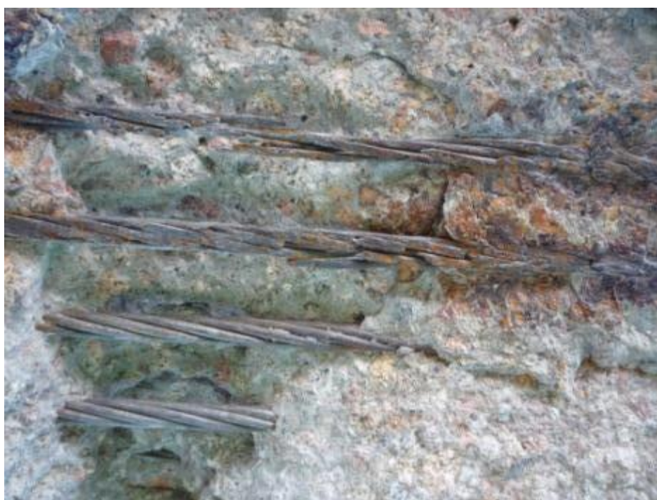
Figure 3 Typical chloride induced deterioration of the prestressed concrete beams
