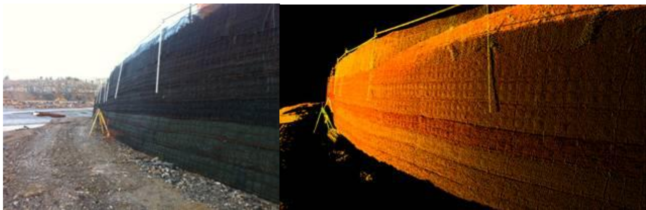
Figure 8. Former Quarry GRS: Photograph (left) and TLS Scanned Point cloud (right) obtained during construction.
