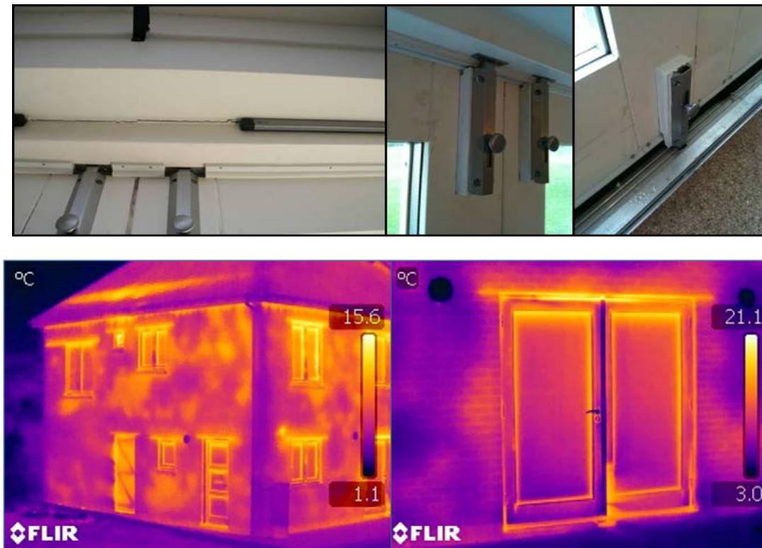
Figure 6 – Observational evidence of poor quality installation and of uneven cavity wall insulation.
