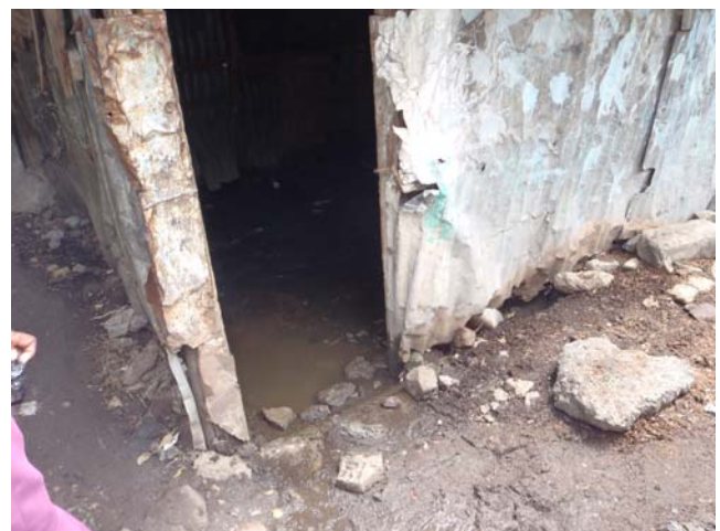
Figure 1. House flooded due to blocked drain, Mukuru, Nairobi, Kenya (photograph: B Reed)
