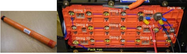
Fig. 10 – String of 6 \times 1.2V 'D' Cells from a Honda 'Insight' battery pack.
