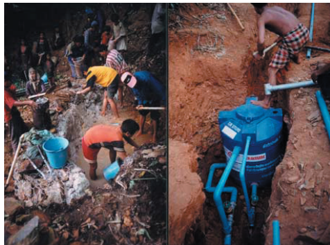
Photograph 2. Building of gabion intake with clay (left) and set up of plastic sedimentation tank (right)
